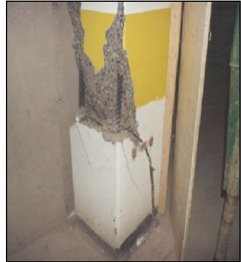
Plate 2: Column failure due to hydrostatic uplift of slab
