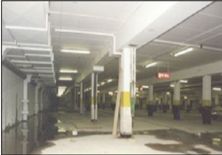
Plate 1: Basement suffering failure due to hydrostatic uplift
